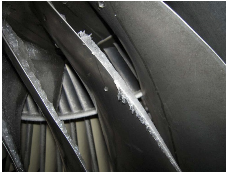
Ice on the Rear Side of the Fan Blades
